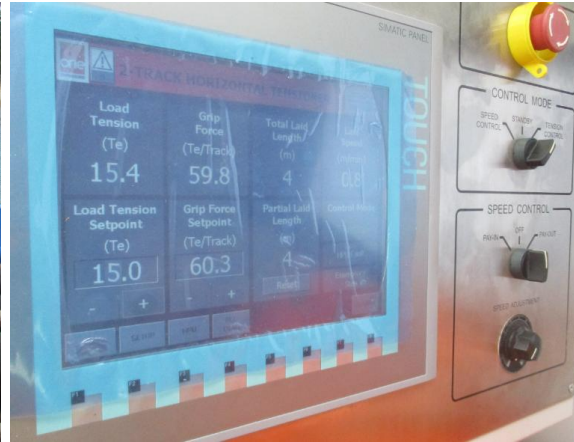
Tensioner Control Console
