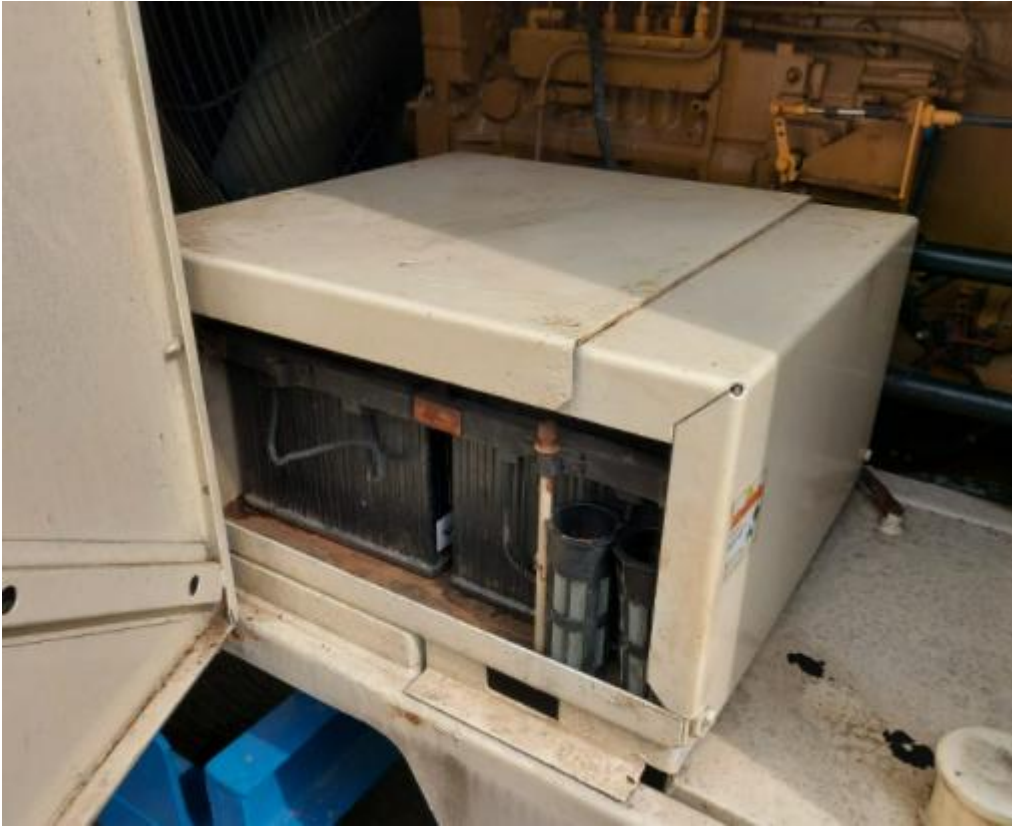
Covered battery isolation
