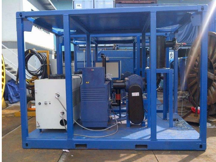
STOKES VACUUM PUMP c/w Booster & Chiller
