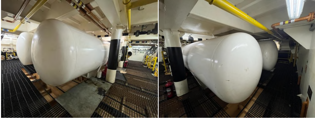
Figure 3-5 Below Deck Air Receivers
