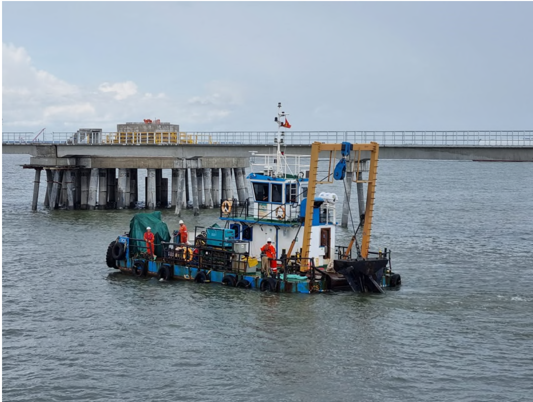
Figure 8-2 Miss Bee Handling 5mT Delta Flipper Anchor in Tra Vinh Wind Farm Installation Project (Vietnam)
