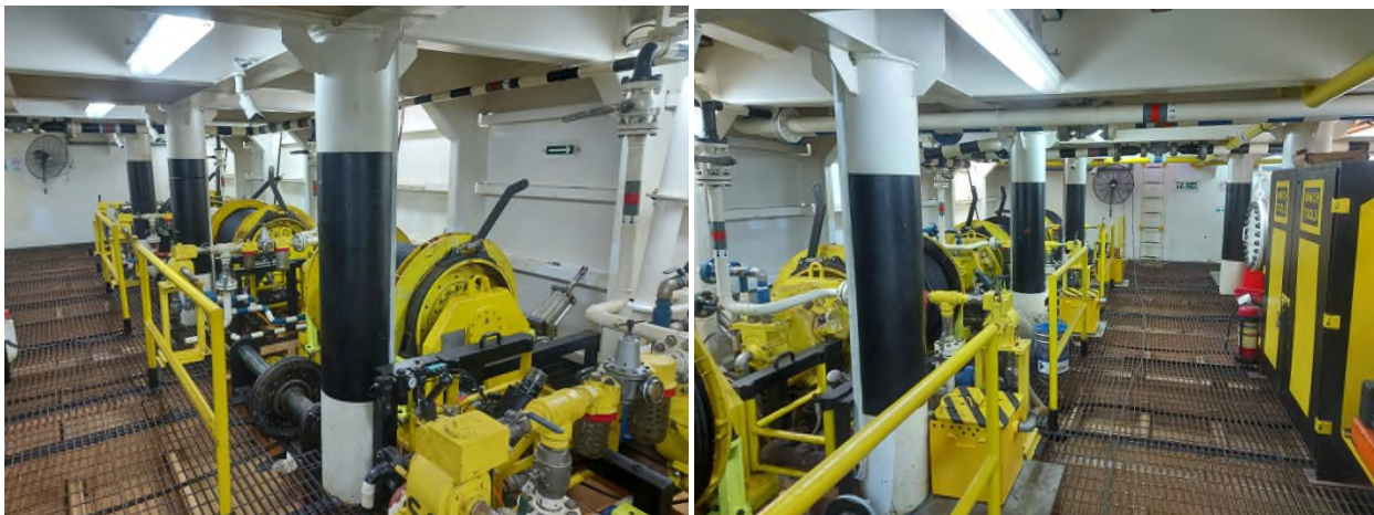
Figure 3-4 8 Nos. 10T Air Driven Mooring Winches (Below Deck)
