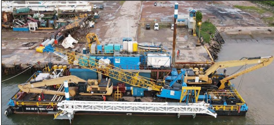
Figure 4-5 UB-01 Loadout – 2x390 Excavators, 1x90T crane, Trailing Arm and Jetting Pumps for Sriracha Project
