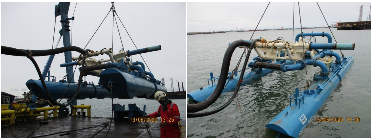
Figure 6-7 Pontoon Articulated Arm function test for project
